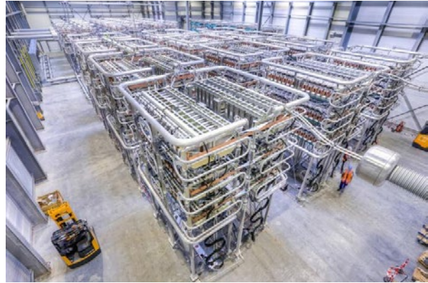
Figure 5: Interior view of a HVDC Plus converter station in Büttel in Schleswig-Holstein, the same technology as will be used for the COBRA converter stations.
